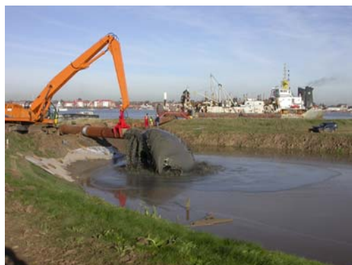
Photograph 9: The mud is pumped into a pipeline and into a retaining bund to settle out
