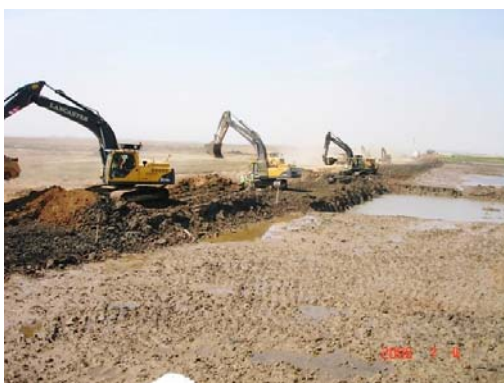
Photograph 3: Final breaching work (8000m 3 of material removed during a 7-hour tidal window)
